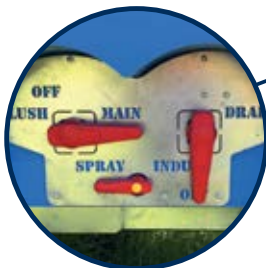
BA control station for spray/flush tank selection or chemical induction tank drain
